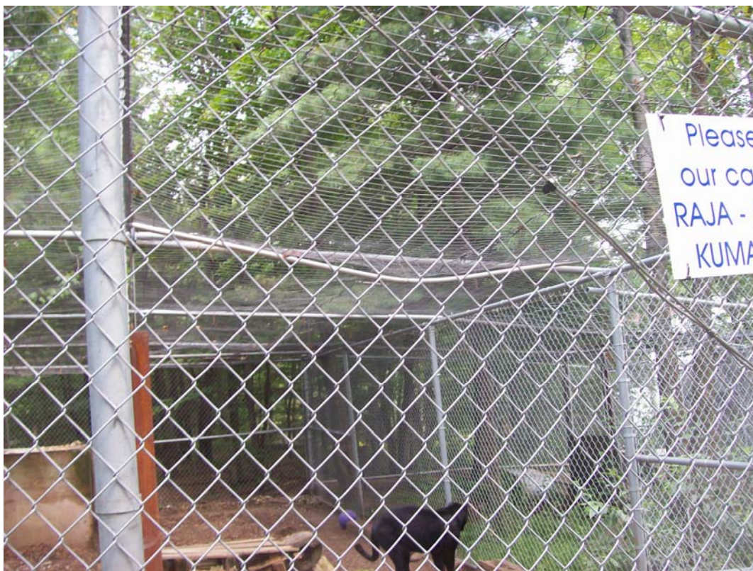
The horizontal ceiling support on this cage should be repaired. All cages must be well constructed and secure, particularly if they contain potentially dangerous animals.
